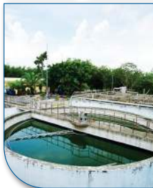
Waste water treatment plant
